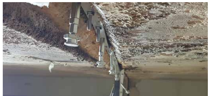
Eingebautes DESOI Quick Seal in einer Fuge | Built in DESOI Quick Seal in a joint
